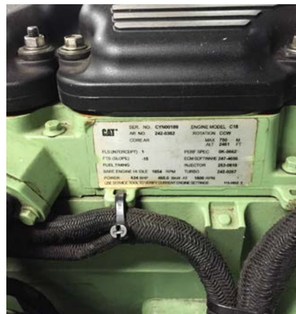
The test is performed on a Catapillar, Type C18 – 624 PS.
